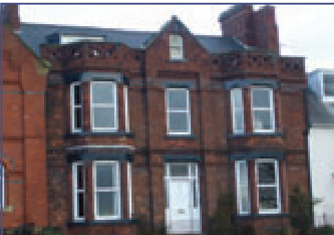
Loss of traditional fenestration, no. 25 The Front
