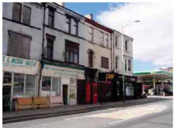
30 21-23 (nearest) High Northgate, with windows boarded up and generally in a poor state of repair, at time of writing, being restored with grant funding.
