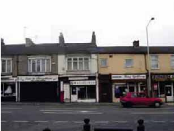
29. Original window and door openings have been replaced, and a poor state of repair prevails (High Northgate).
