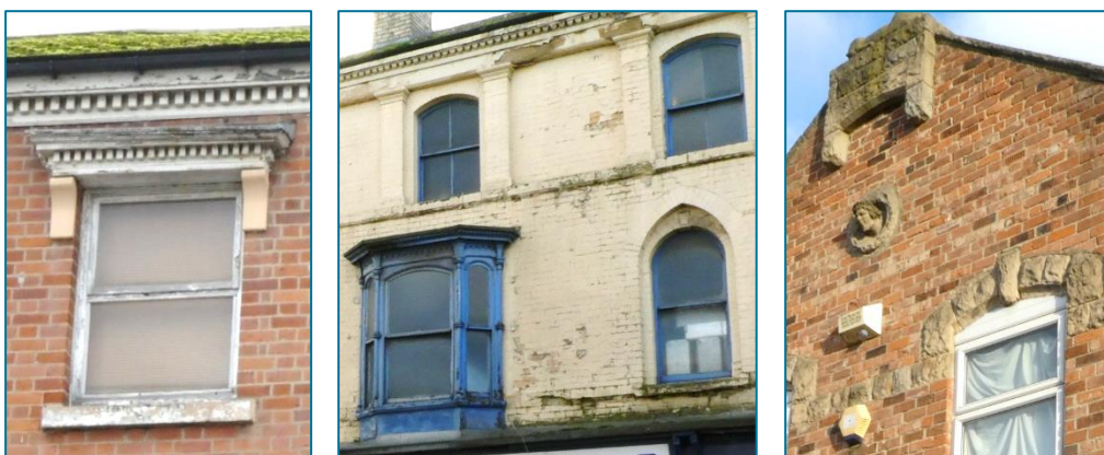
Left: Brick building with Italianate stone detailing to eaves and canopy above window. Centre: [E] Livingstone Building – All walling and detailing in brick, later painted; decorative bay window constructed in timber. Right: [F] 1 Leadenhall Street – Distinctive stone carvings by Robert Borrowdale (Photos © Gaby Rose, 2023)
