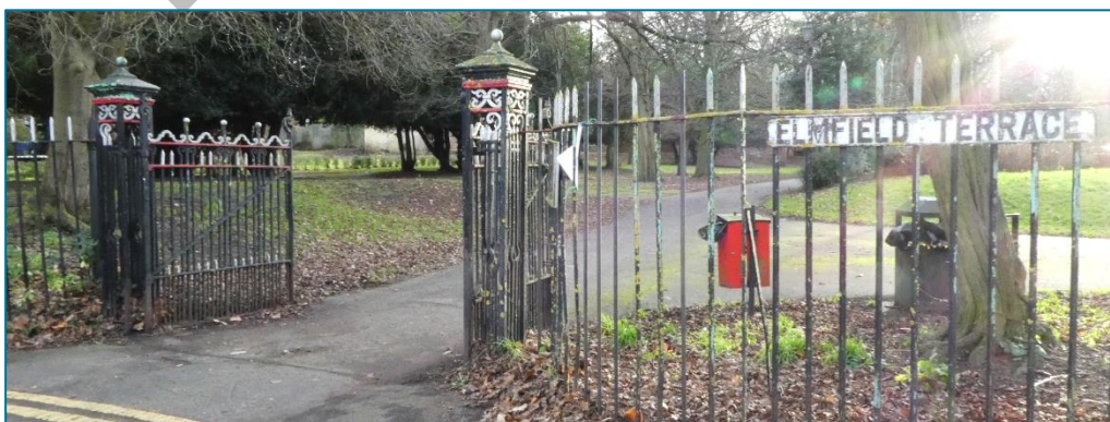
Original cast-iron railings and gate piers to North Lodge Park. (Photo © Gaby Rose, 2023)
