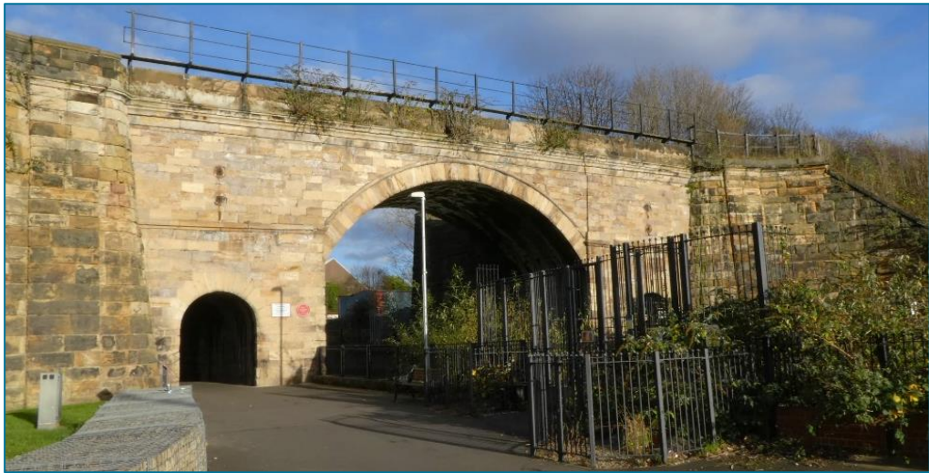
[7] Skerne Bridge (photo © Gaby Rose, 2023): Railway bridge designed in a classical style by Ignatius Bonomi for the S&DR, 1825; subsequently altered/strengthened. It is the only architect-designed bridge on the S&DR 54 and featured on the company's headed paper. Now the world's oldest railway bridge still in use.
