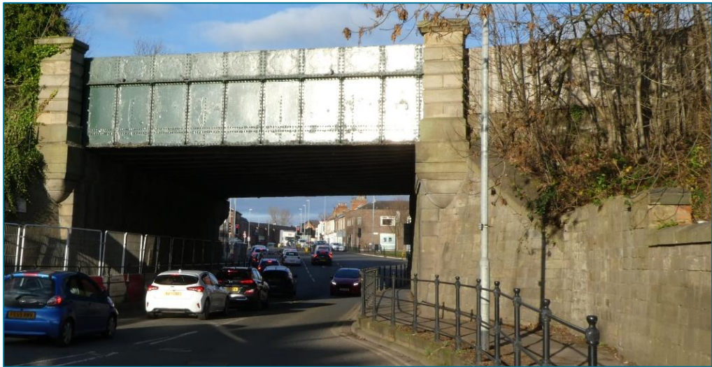
[6] Railway Viaduct (photo © Gaby Rose, 2023): Plans to build a bridge were begun in the 1840s, and the bridge finally built in 1856; altered/rebuilt in 1876, and road level further dropped after 1949 to allow for double-decker busses 102 . An early photograph shows a plaque with the date MDCCCLVI on the side. Altered prior to 1935.
