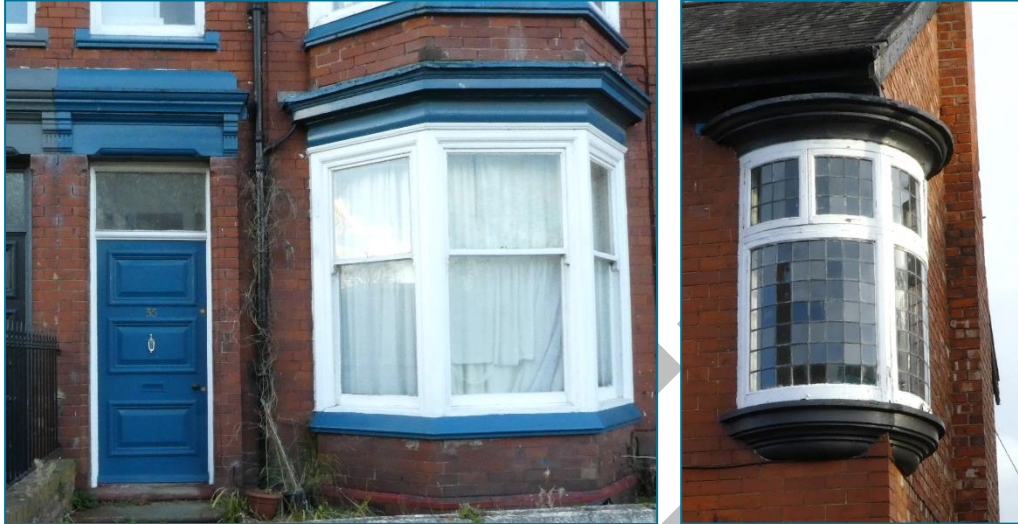
Left: Original panelled door with stone canopy over and old windows along North Lodge Terrace. Right: Curved first-floor window along Elmfield Terrace (Photos © Gaby Rose, 2023)
