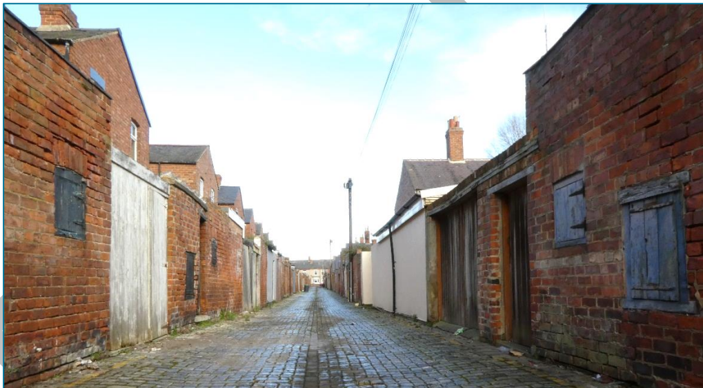
Back lane to rear of North Lodge Terrace, looking north; note the original shuttered openings to both sides. The rendered wall further on to the right has a harmful impact on the historic character of this lane. (Photo © Gaby Rose, 2024)
