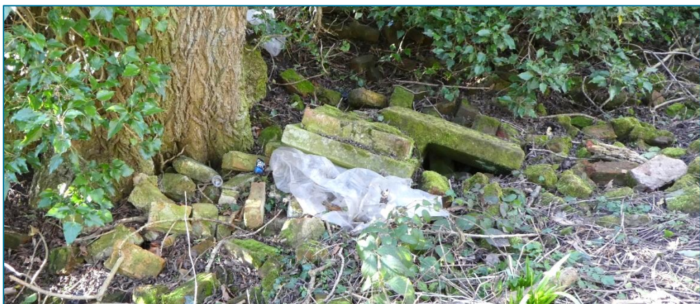
Top: End section and terminal pier (right) of former reservoir embankment walling that has been destroyed by vandals. Bottom: Discarded rubbish, bricks and stone cappings opposite the dismantled walling. (Photos © Gaby Rose, February 2025)
