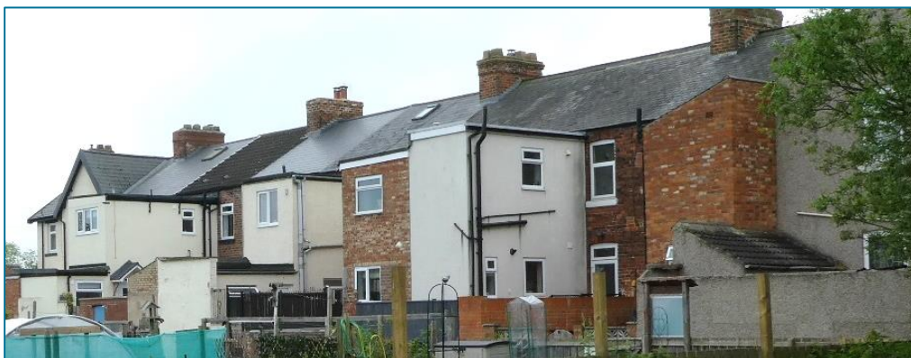
Extensions to rear of traditional terrace with flat roofs, modern renders and inappropriate window proportions, viewed from public footpath. (Photo © Gaby Rose, May 2024)
