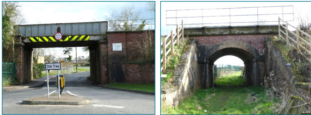
Left: [S] Metal Railway Bridge over the historical route to Yarm. Right: [R] Masonry Railway Bridge over access track. (Photos © Gaby Rose, March 2024)
