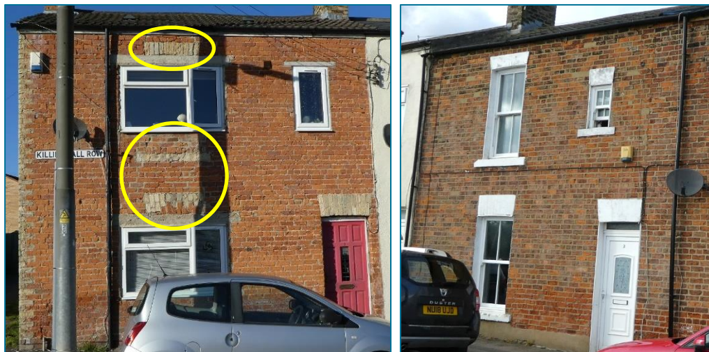
Left: The northern end house of Killinghall Row shows that, despite the insertion of larger openings, the original lintels have been retained (circled in yellow). This is likely to be the case with many of the other properties that have been altered. The reinstatement of the original openings here should therefore be fairly straightforward (Photo © Gaby Rose, February 2025). Right: Cross references can be made by looking at properties within the row that have been well preserved. Here, the replacement frames using a 2x2 sash type seems appropriate for the construction date of the row (c.1864). Note that these are uPVC windows which is not evident unless you look in detail! Their slim frames and glazing bars as well as them being set back in the masonry allow them to fit in almost perfectly (Photo © Gaby Rose, March 2024).
